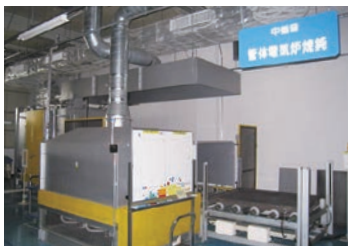
Reduction in power consumption at a Japanese factory through update of an electric annealing furnace
