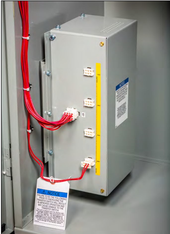
Figure 6. Voltage Selection Terminals.
