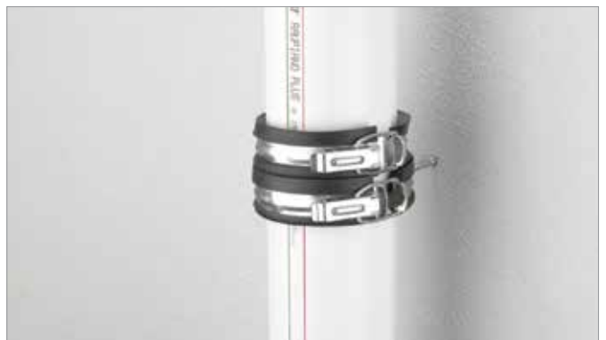
Fig. 7-17 Fully installed sound-dampening bracket.
