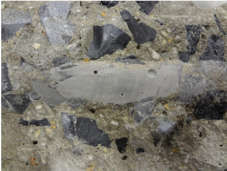
(Figure 4 – Exposed adhesive anchoring material indicating no bond to cement concrete)
