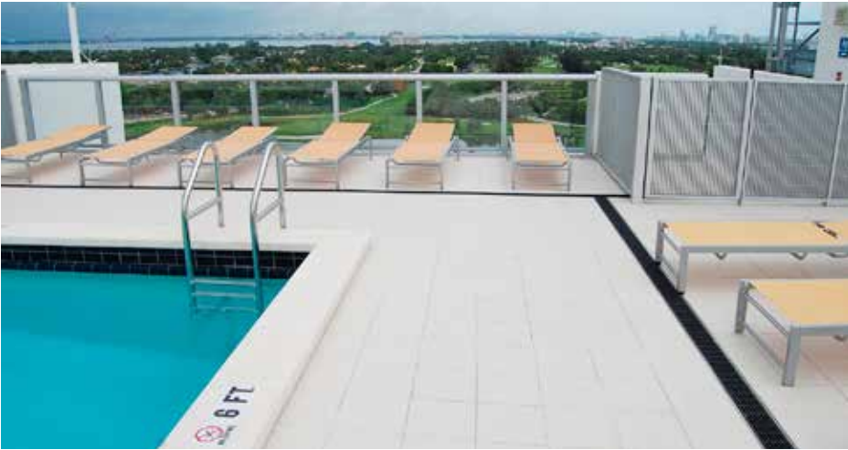
Stainless steel was specified for this pool because it is long-lasting, does not harbor bacteria, and can stand up to pool chemicals. A ductile iron grate was selected to prevent bathers from slipping.
