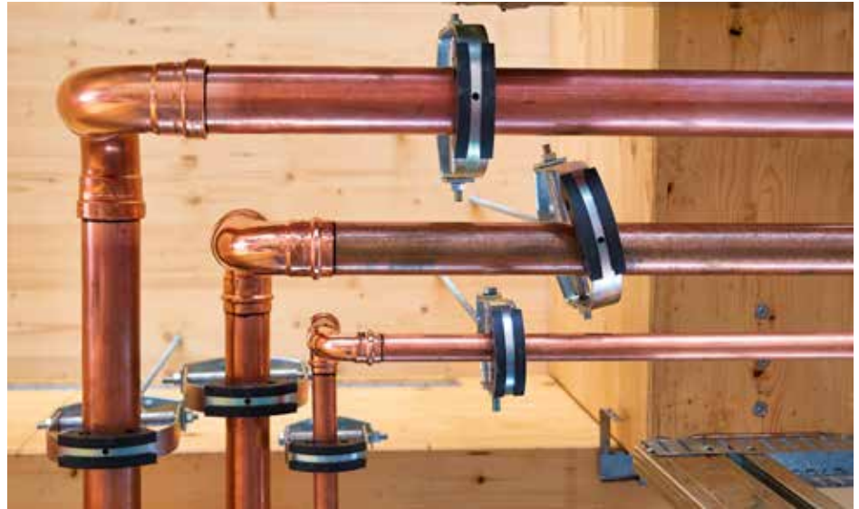
Viega's two new buildings use ProPress fittings behind the walls to provide potable water because, as Braconier President Tom Stone said, soldered joints might leak, but ProPress joints do not.
