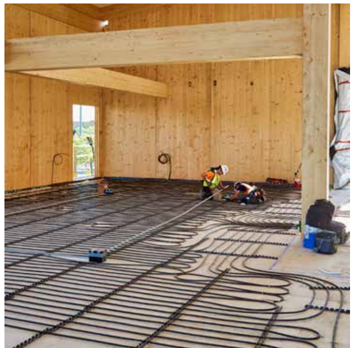
The radiant system in the seminar center—which contains more than 36,000 linear feet of tubing—was the largest Braconier had ever installed. The bare concrete floors stay comfortable year-round with the radiant products.
