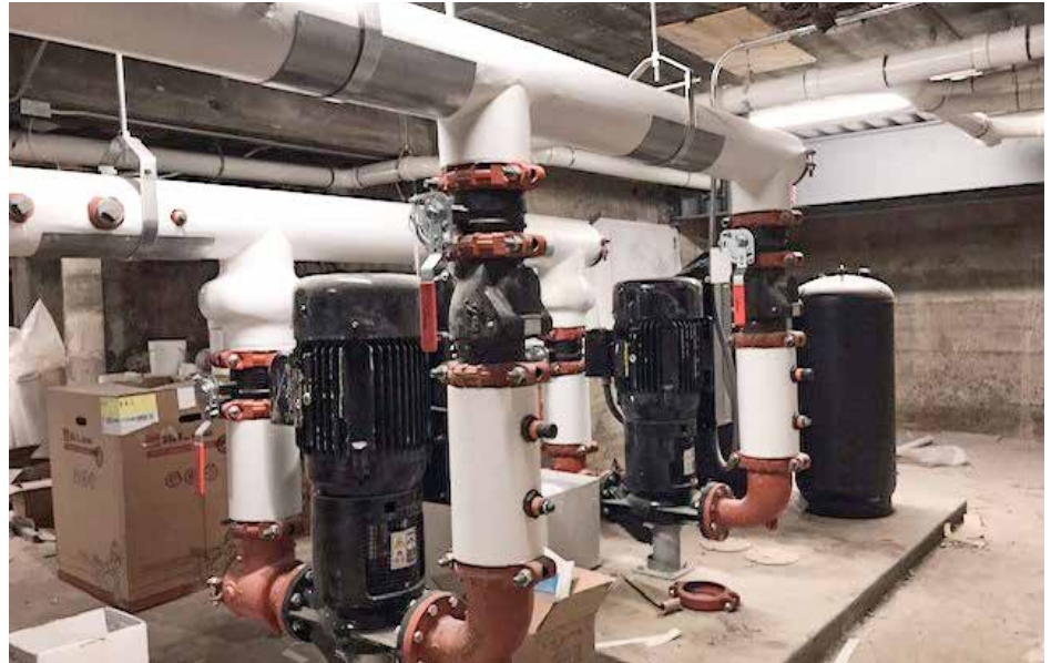
Collaborating with Victaulic's Virtual Design and Construction team to use BIM to schedule the work resulted in significant time savings, allowing Kruse installers to complete 80 percent of the basement in just a few days.
