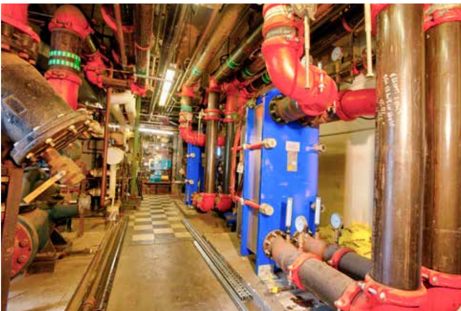
Replacing the Benjamin Franklin House's old cooling tower with a modernized version allowed for minimal pipework, saving Elliot-Lewis time.
