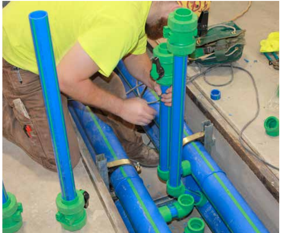
Warner Mechanical found that Aquatherm polypropylene pipe was ideal for the new IVP Plastics facility, and it is easier and faster to install than traditional welded pipe, saving the contractor time and money.
