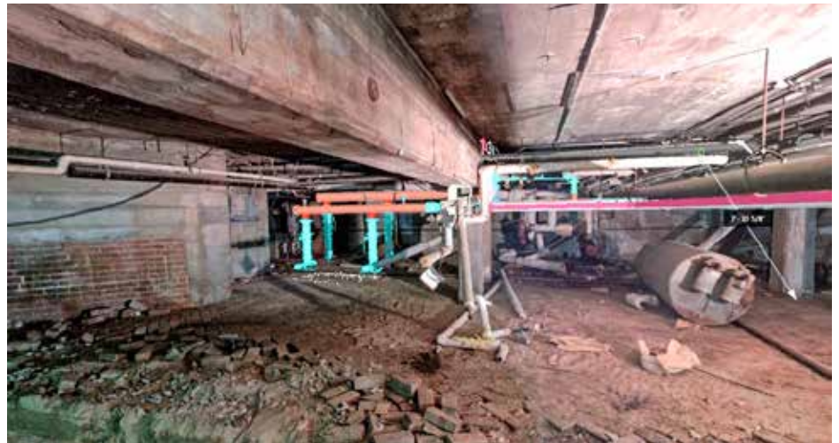
Victaulic's 3D scans streamlined design conversations with Kruse and others, because the model and the scans could be overlaid to ensure the designs were aligned with the space.
