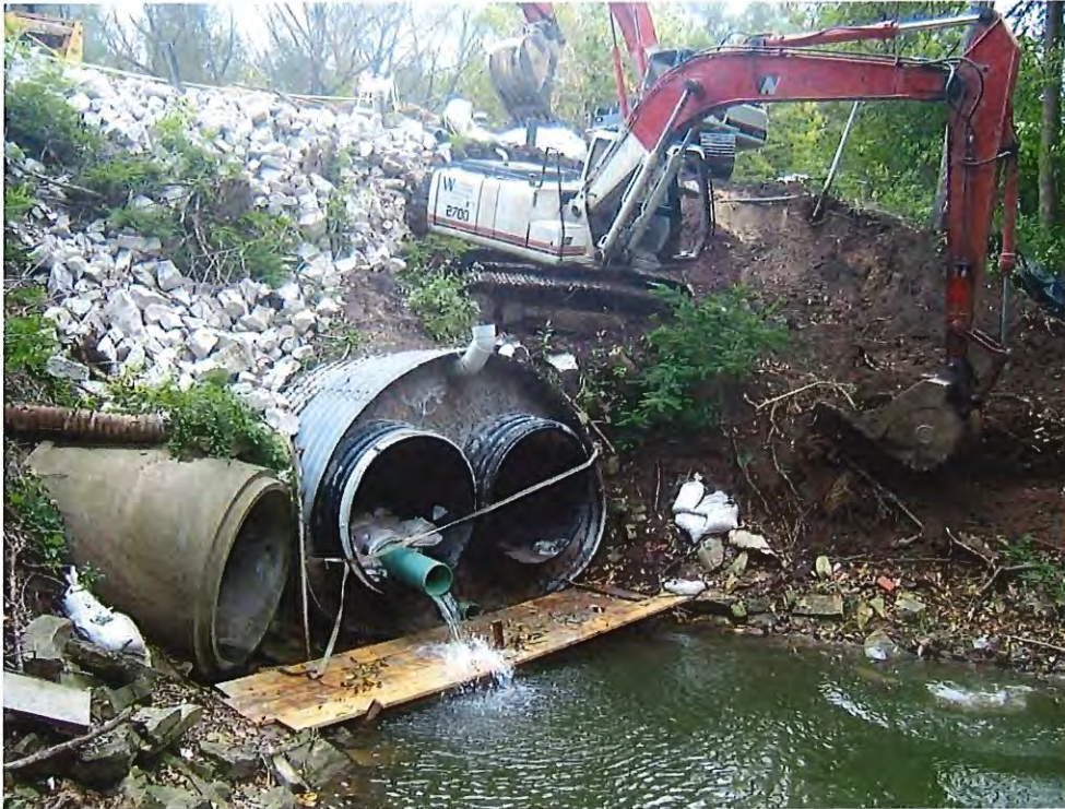
Figure 7.1 – The County Line Road culvert replacement project was completed with joint effort between the City of Mequon and the Village.
