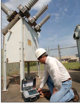
The S1-552/2 in use at an industrial complex substation
