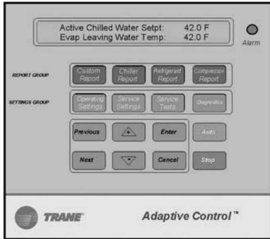
Figure 35 Operator Interface Adaptive Control
