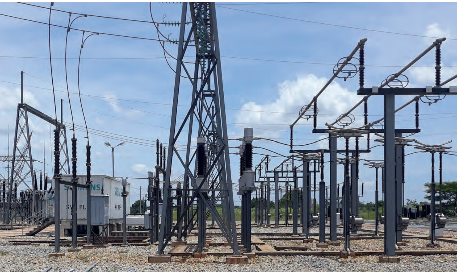
Mocuba substation in Mozambique
