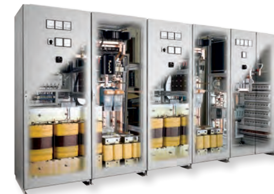
400kW aircraft engine test, 290V DC power supply system, dual 700A configuration for highly inductive load (turbine)
