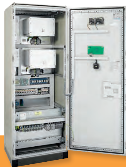
Hydroelectric power station, redundancy n+2
