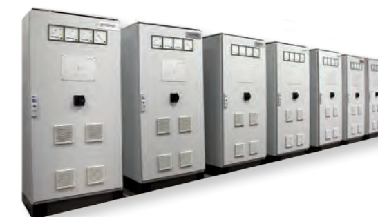
DC power 200kW for the airport, 110 VDC power generation, dual 800 A configuration, full load operation up to +55 °C ambient temperature, protection degree IP42
