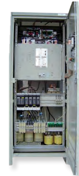
UPS System in a cabinet
