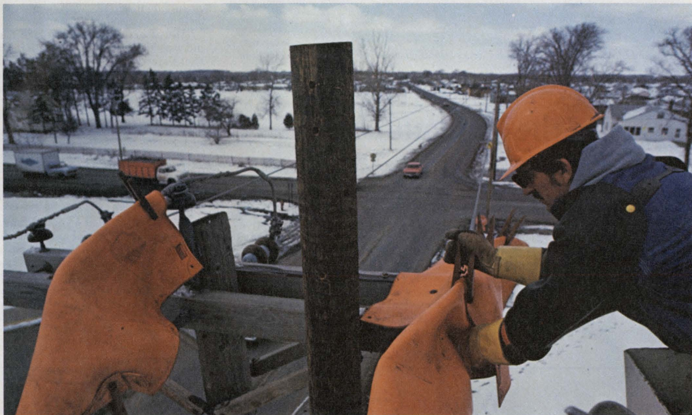
To increase the power available to customers in Fridley, Minn., a Northern States Power Co. construction crew is converting a single-phase 13,800-volt line to three-phase service.
