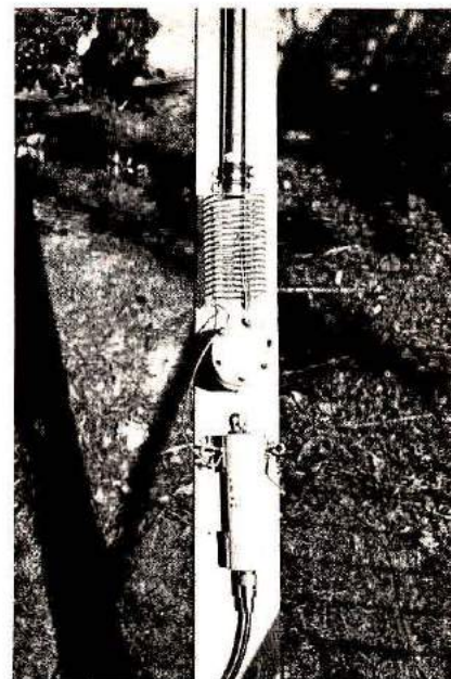
A plumber's delight with balun and matching coils can be mounted on a piece of board before it is fastened to the end wall of a house.
