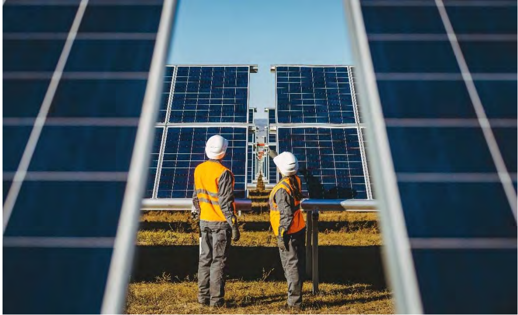
Figure 3-11: Representative Photo of Single-Axis Tracking PV System in the Morning, Facing East
