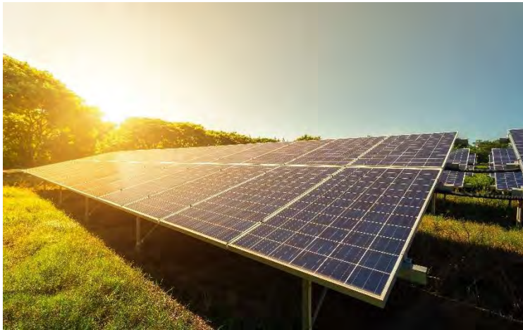
Figure 3-12: Representative Photo of Single-Axis Tracking PV System at Midday, Laying Flat
