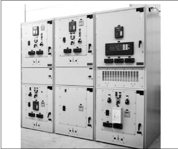
Figure 1. Example of an ANSI/NEMA Assembly
