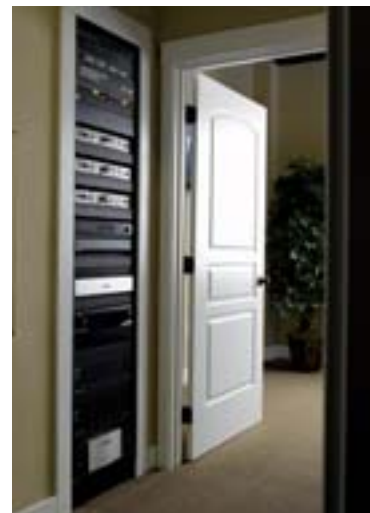
Above: The media closet stores all your home automation gear, allowing you to keep everything hidden and in one location.
