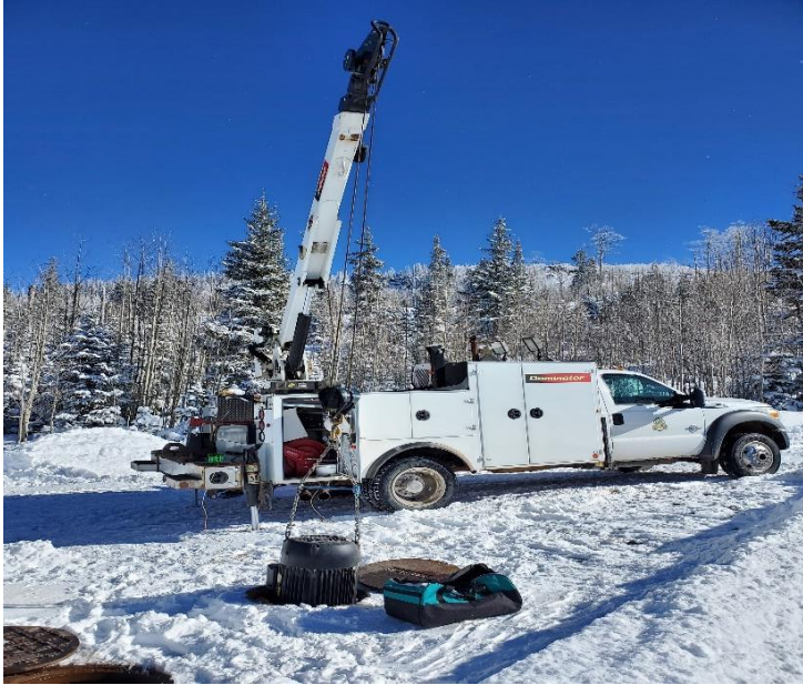
Using the new service truck to install a motor at snowflake booster station
