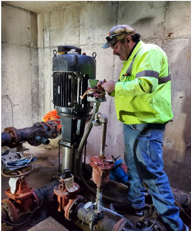
Chris wiring up the Motor taken from Million Gallon Pump Station and installed into Snowflake Booster
