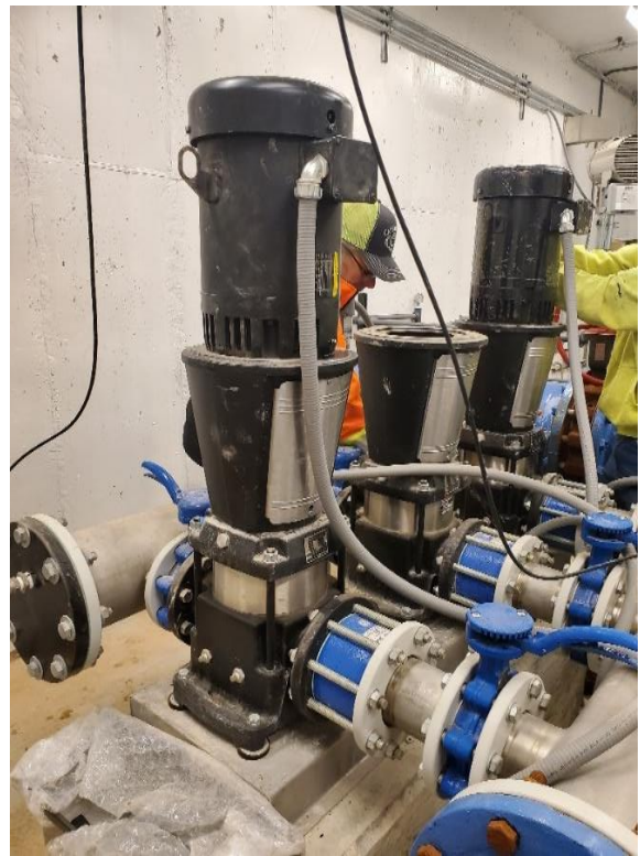
Operators performing maintenance on motors in the Mammoth Pump Station
