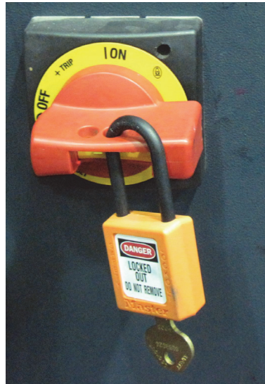
Figure 1-2 Lock-out of the Main Power Switch
