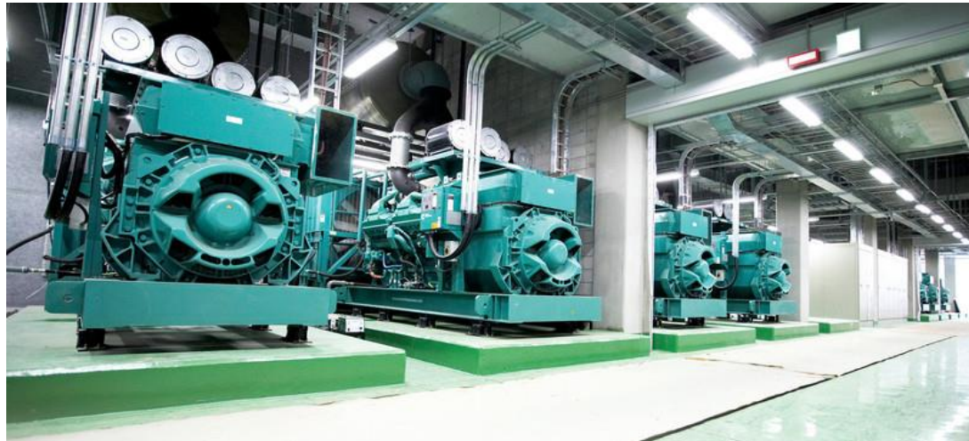
Standby power system including seven C2000 D6 (2000 kWe) generator sets.
