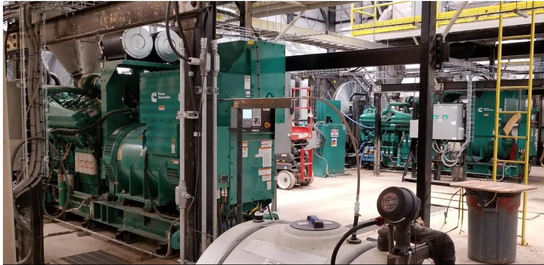
Remote mining site including two DQGAS (1500 kWe) generator sets.
