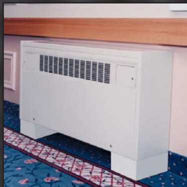
Cabinet Unit Heaters
