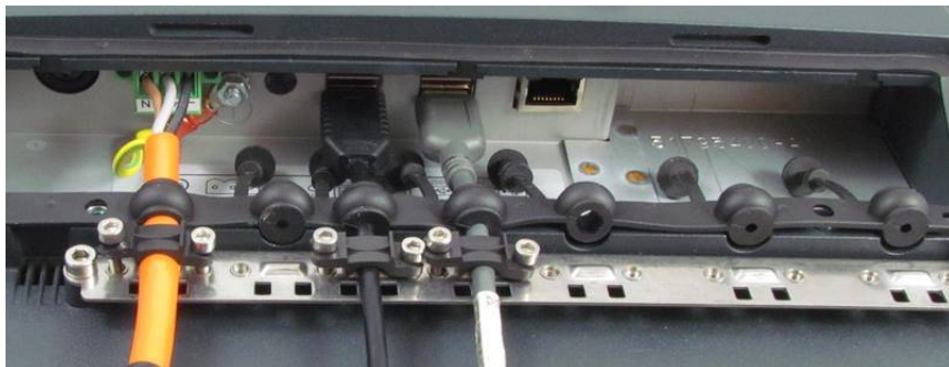
Fig. 8.5: USB cable on the connector panel; secured to the strain relief rail
