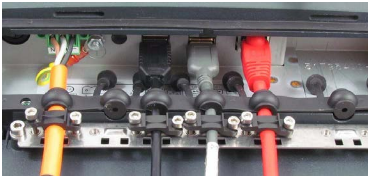
Fig. 8.6: Ethernet cable on the connector panel; secured to the strain relief rail
