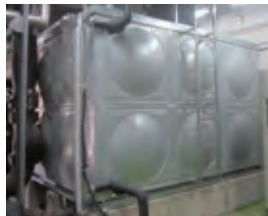
Tank that stores drain water
