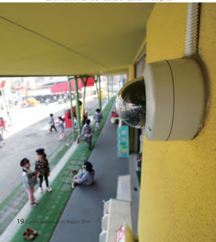
Canon network camera installed at Yayoidai Kindergarten
