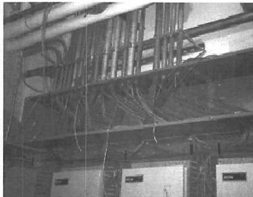
Feeder Tubes, Cables, and Junction Box
