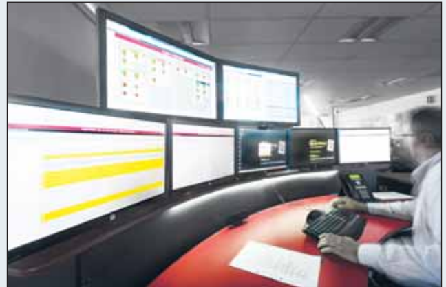
Siemens' Smart Grid solution for Maharashtra State Electricity Distribution Corporation Ltd. will reduce transmission and distribution losses in eight cities.
