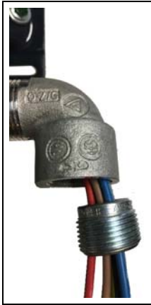
Figure 12: Bushing inside the Elbow Joint
