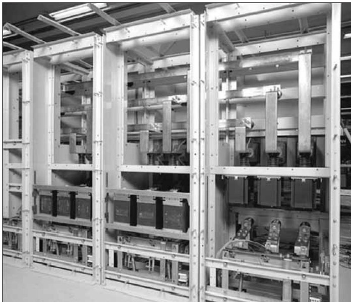
Figure 14. Internal View of Typical Sections of an IEC Metal-Enclosed Switchgear (No Barriers Between Sections, nor Busbars Covered by Insulating Materials)
