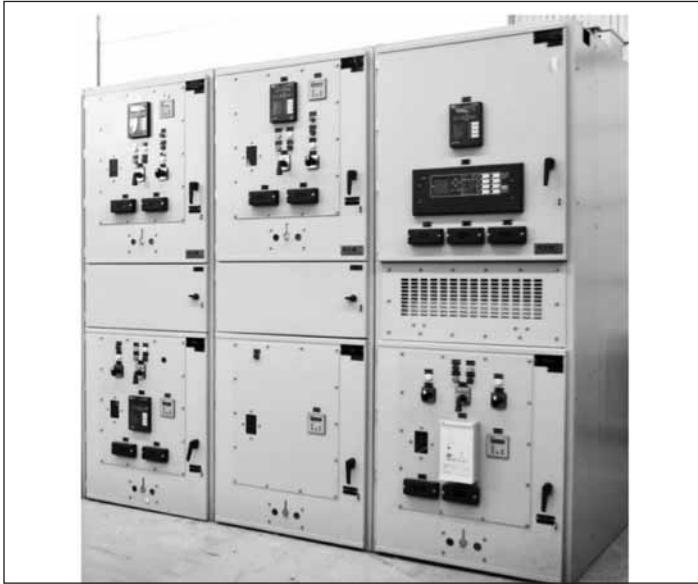
Figure 1. Example of an ANSI/NEMA Assembly
