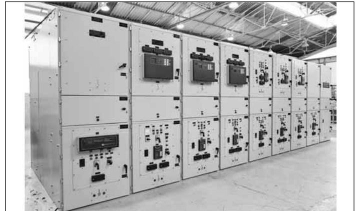
Figure 4. MV Switchgear Assembly Corresponding to the Single-Line Diagram Shown in Figure 3
