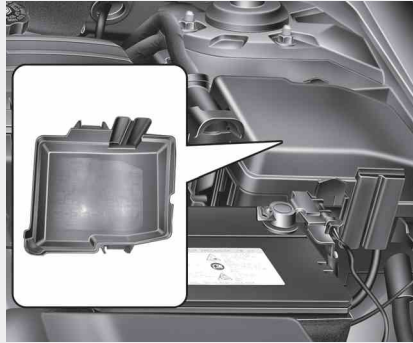
Engine compartment fuse panel
