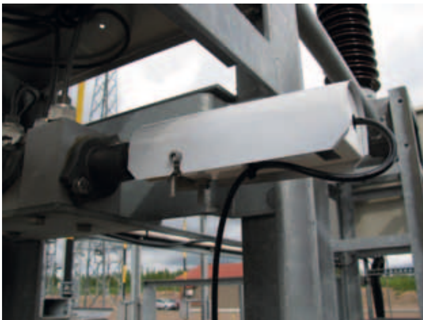
Outdoor installation into a "sensor block".
