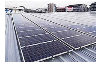
Solar panels on the roofs of some Kanagawa Nissan dealerships. Power from the panels is supplied to dealerships through the PPS system.
