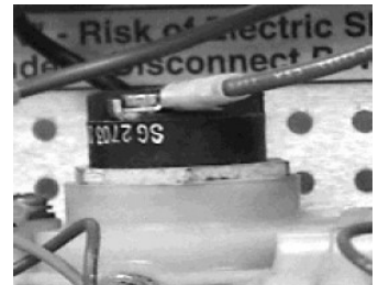
Figure 11: Installed heating element
