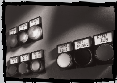
Labeling of push-buttons and signal lamps
