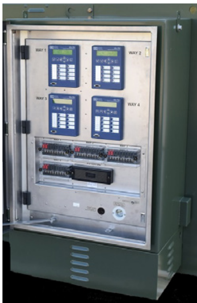
Figure 17. Schweitzer Engineering Laboratories Multiple SEL-751's integrated in exterior cabinet.
