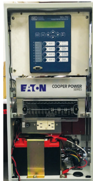
Figure 18. Schweitzer Engineering Laboratories SEL-751 integrated in internal cabinet.
