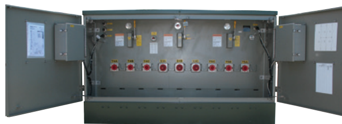
Figure 2. VFI switchgear 6-way unit.
