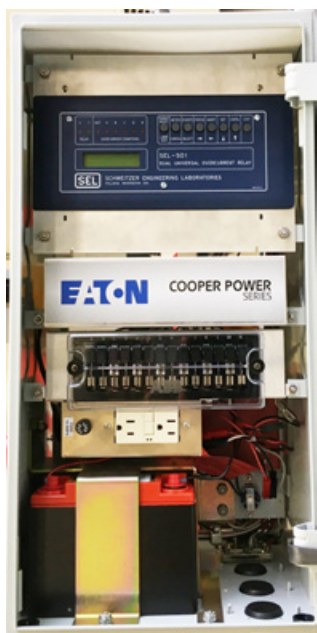
Figure 19. Schweitzer Engineering Laboratories SEL-501 integrated in cabinet.
