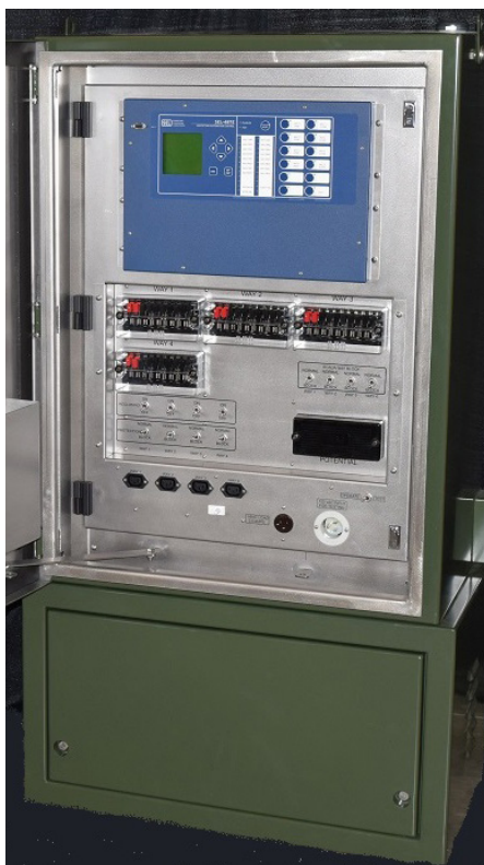
Figure 23. Schweitzer Engineering Laboratories SEL-487e integrated in exterior cabinet.
