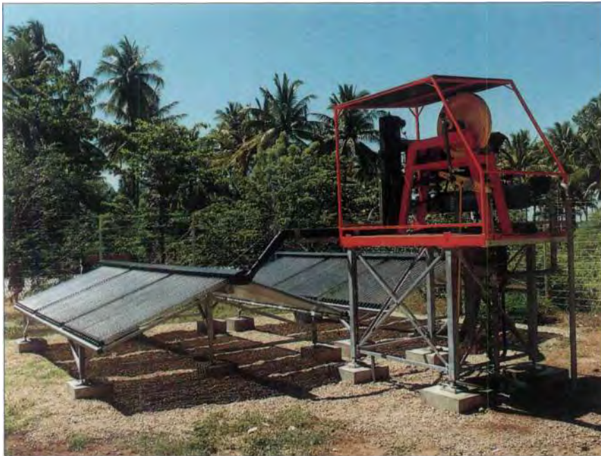
Dornier has conducted projects using regenerative energies in 18 countries in the Third World. This picture portrays a solar-powered drinking water pump in Indonesia.
