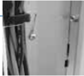
Figure 55: Communication Ground Termination 2
