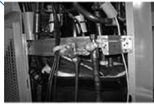
Figure 58: Refrigerant Pipe Connection Point 1
