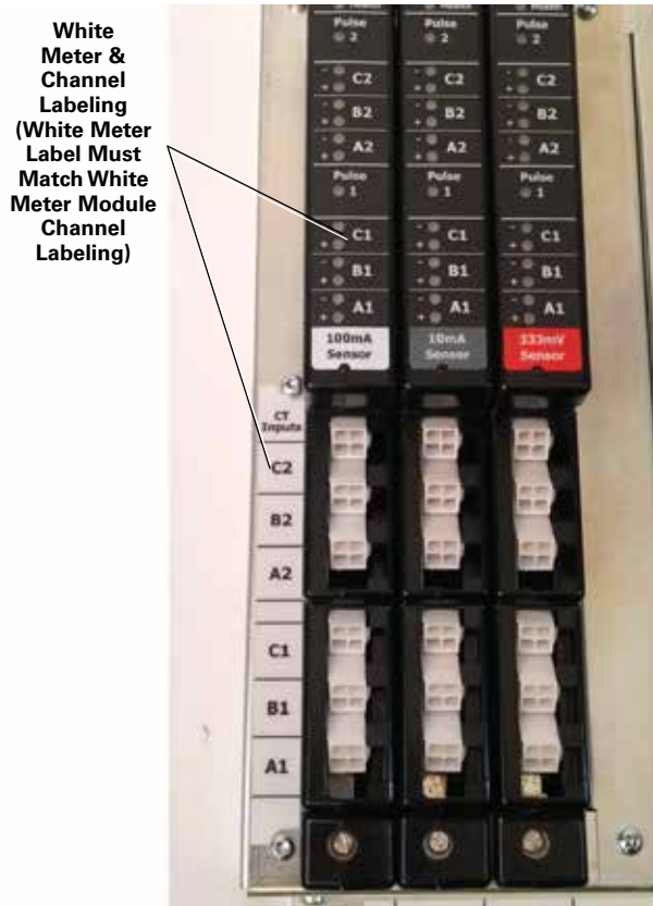
Figure 12. Phase Assignment Label: PXMP-MB Assembly. Note Matching Black/White Meter Base and Meter Module Lens Phase Markings.
