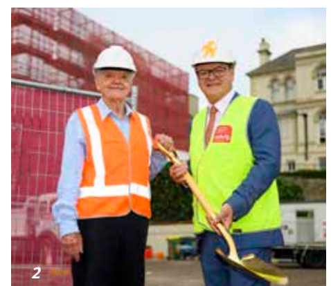
when Stage 1 of the construction of the John Cunningham Student Centre commenced in January.
