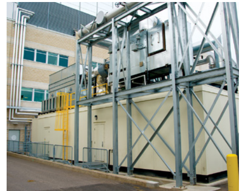
The CHP plant produces more than 16 million kWh of power and around 50 billion BTUs of heat per year.
