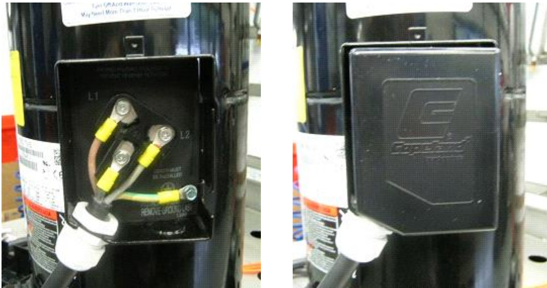
Figure 20: Correct electrical installation with cable glands for IP21 T-box (compressors ZBD30K* to ZBD114K*, ZFD13KVE to ZFD25KVE & ZFD41K5E)
