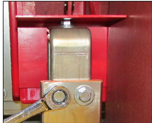
Fig. 44 Checking Power Fuse Clamping Bolt Torque
