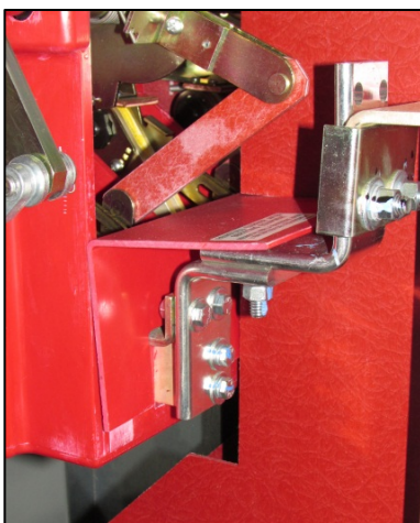
Fig. 46 Angled Barrier In Front Of The Isolation Switch
