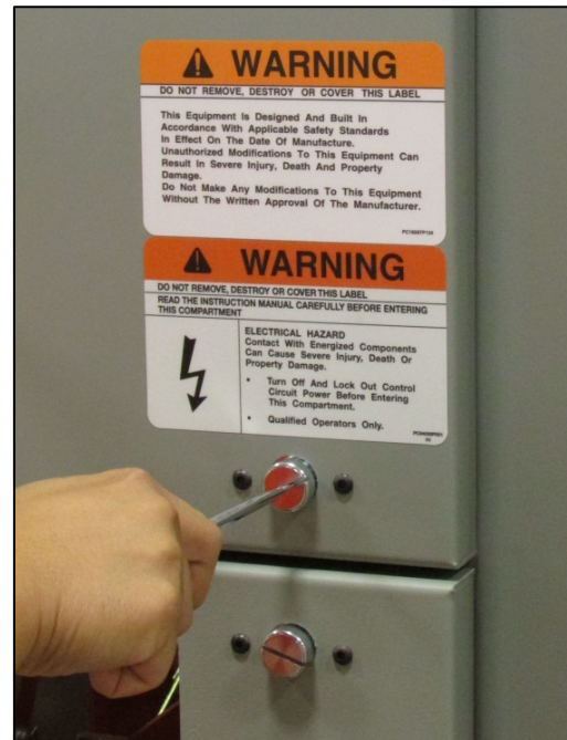
Fig. 38 Preparing For Initial Energization
