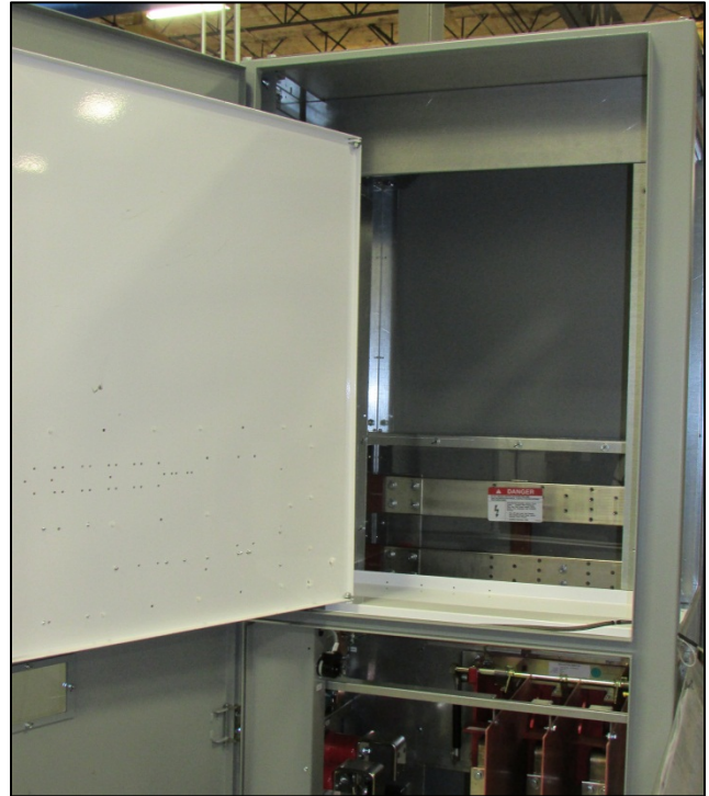
Fig. 35 Low Voltage Subpanel Opened to Expose Main Bus
