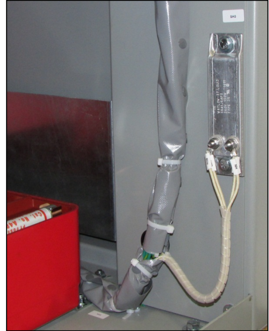
Fig. 5 Typical Space Heater
