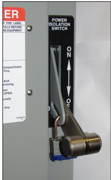
Fig. 24 Isolation Switch Lockout
