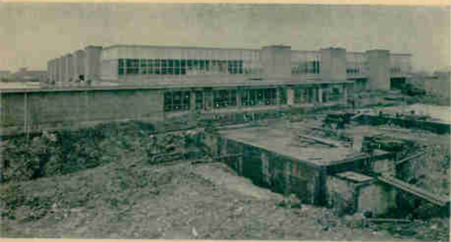
Texas Instruments' new plant at Bedford, England
