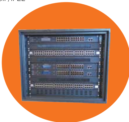
INSTRUMENT ROOM 9U PHONTECH SYSTEM CABINET
