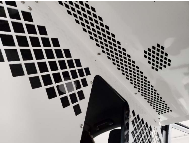
Attach ceiling to bulkheads with 1/4" x 3/4" Phillips head bolts and flat washers.
