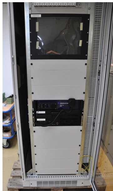
19" Cabinet for weather system
