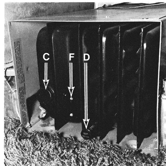
Furnace Controls (21 Ft.)
