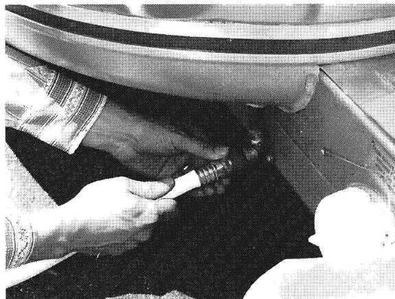
City Water Hook-Up
