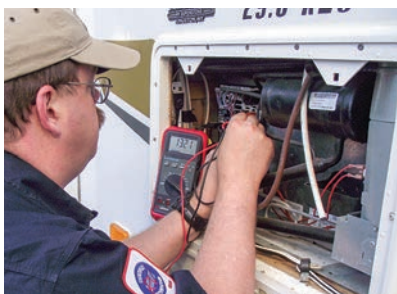
An RV refrigerator requires 12-volt DC, 120-volt AC or propane gas to heat the cooling unit, and 12-volt DC to operate the electronics at all times. Having the correct gas pressure and electrical supply coming into the unit are essential for proper operation.
