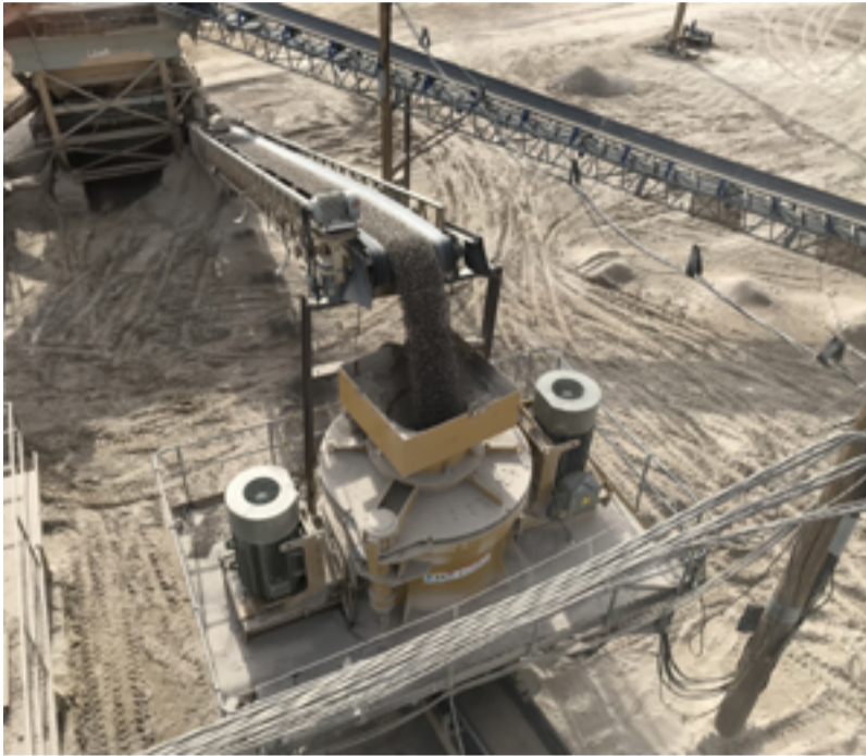
Figure 2: Vertical Shaft Impact Crusher The dry process vertical shaft impact crusher uses twin 400 hp motors to crush 1.5-inch rock to 1/8-inch minus sand that is fed to the wet plant.
