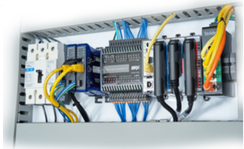
Figure 2: VPN cabinet. By only providing the functionality needed for IIoT connectivity, this AutomationDirect StrideLinx VPN router, installed on the far right of the DIN rail and connected to the PLC, simplifies implementation and use.
