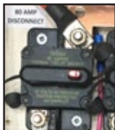
80 Amp Charger Input Breaker
