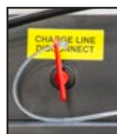
Charge Line Disconnect (red key)
