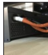
Inverter DC Output
