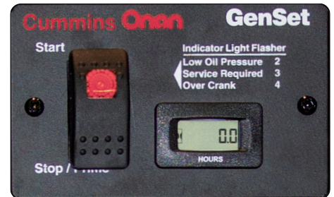
On the G-Class the Generator Remote switch is found on the Command Center
