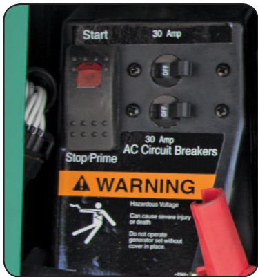
Generator main power & circuit breaker switches.
