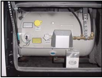
Figure 3-4. Liquid Propane Tank
