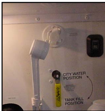
Figure 11-8. City Water Connection
