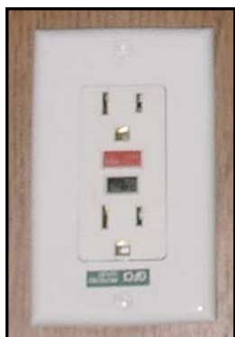
Figure 7-11. Ground-Fault Circuit Interrupter (GFCI)
