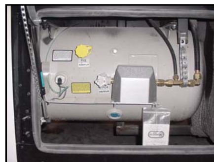
Figure 2-4. Liquid Propane Tank
