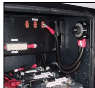
Figure 7-7. Rotary Switch to Disconnect “House” Batteries
