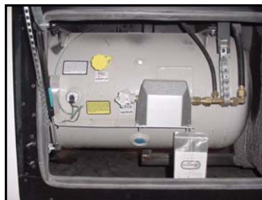
Figure 2-3. Liquid Propane Tank
