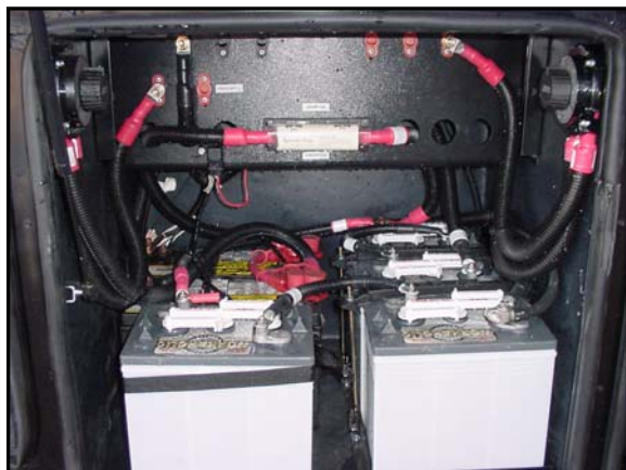
Figure 7-5. 12 VDC Battery Supply (Compartment)
