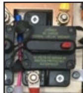
80 Amp Charger Output Breaker
