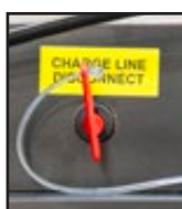
Charge Line Disconnect (red key)
