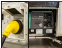
Shore Power or Generator
