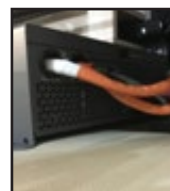
Inverter DC Output
