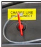
Charge Line Disconnect (red key)
