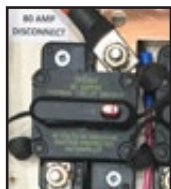
80 Amp Charger Input Breaker
