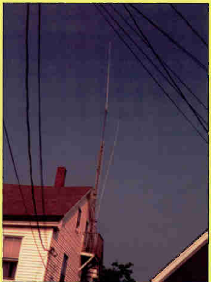
Here's a shining example of a poorly-maintained tower. It's completely rusty and has been erected too close to metal objects, including power lines. It's a disaster waiting to happen.
